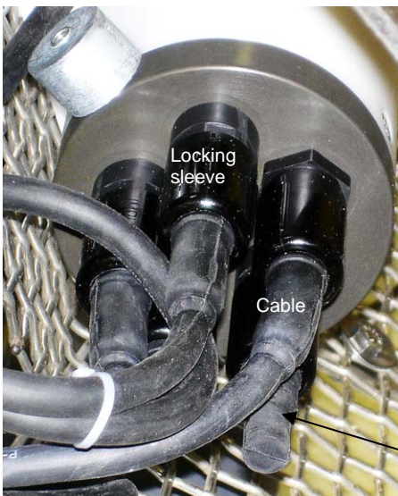
Electronics Control Module shown; verify dummy plug or cable installed for every connector on ECO and CTD
